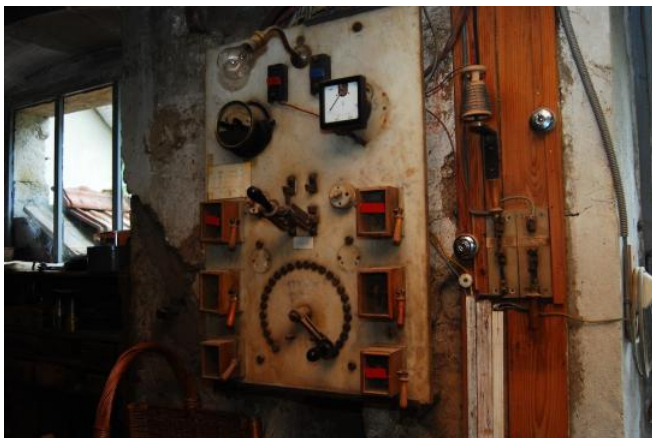
Old Electrical Control Panel
