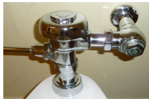
Misaligned Sloan Valve
